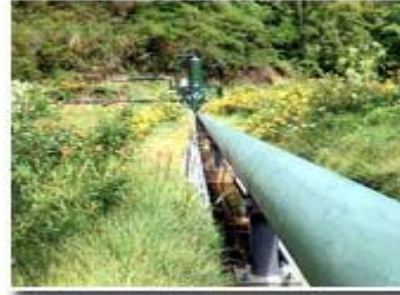
water pipe from production well
